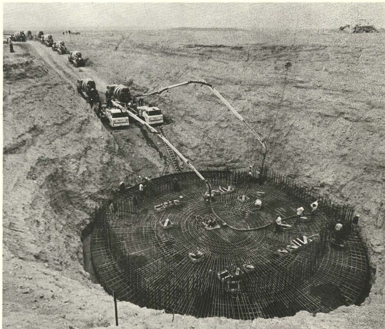
GETTING to the base of things, concrete trucks line up for a 14-hour pour for the foundation of the 5 MW Solar Thermal Test Facility — the "Power Tower." The concrete tower will rise 200 feet above the Coyote Canyon mesa. Several hundred heliostats will focus solar radiation on receivers located on top of tower.
